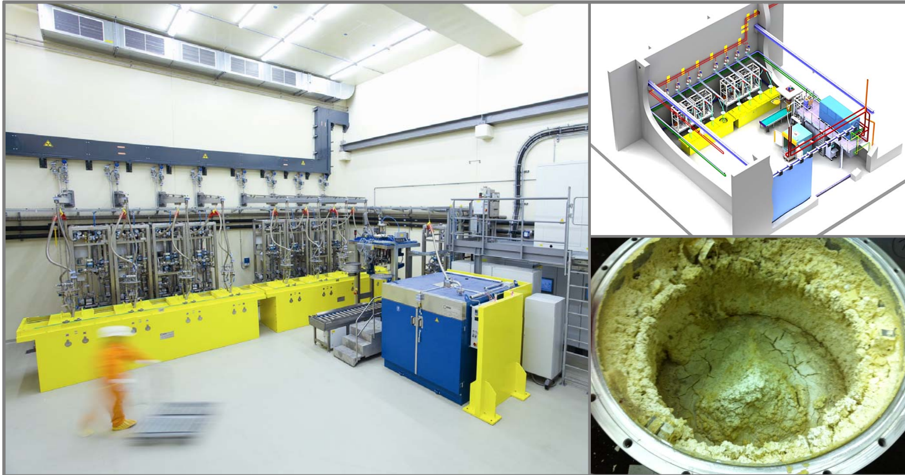
Eight Leg In-Drum Drying Facility for Evaporator Concentrate incl. Infrastructure
